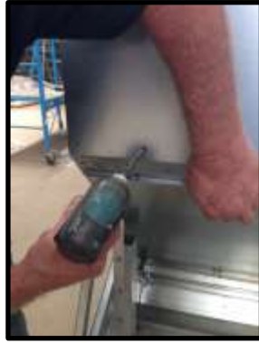
STEP 62: Second tek screw to be the second hole from the end (Do not do the hole at the end first).
