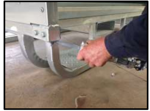
STEP 75: Tighten fully bolts and nuts connecting posts to base. Sealastic the bottom of the posts to the frame. Ensure water tight.
